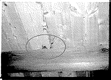
Photo: 7000 Stain noted in the kitchen on ceiling (1)
